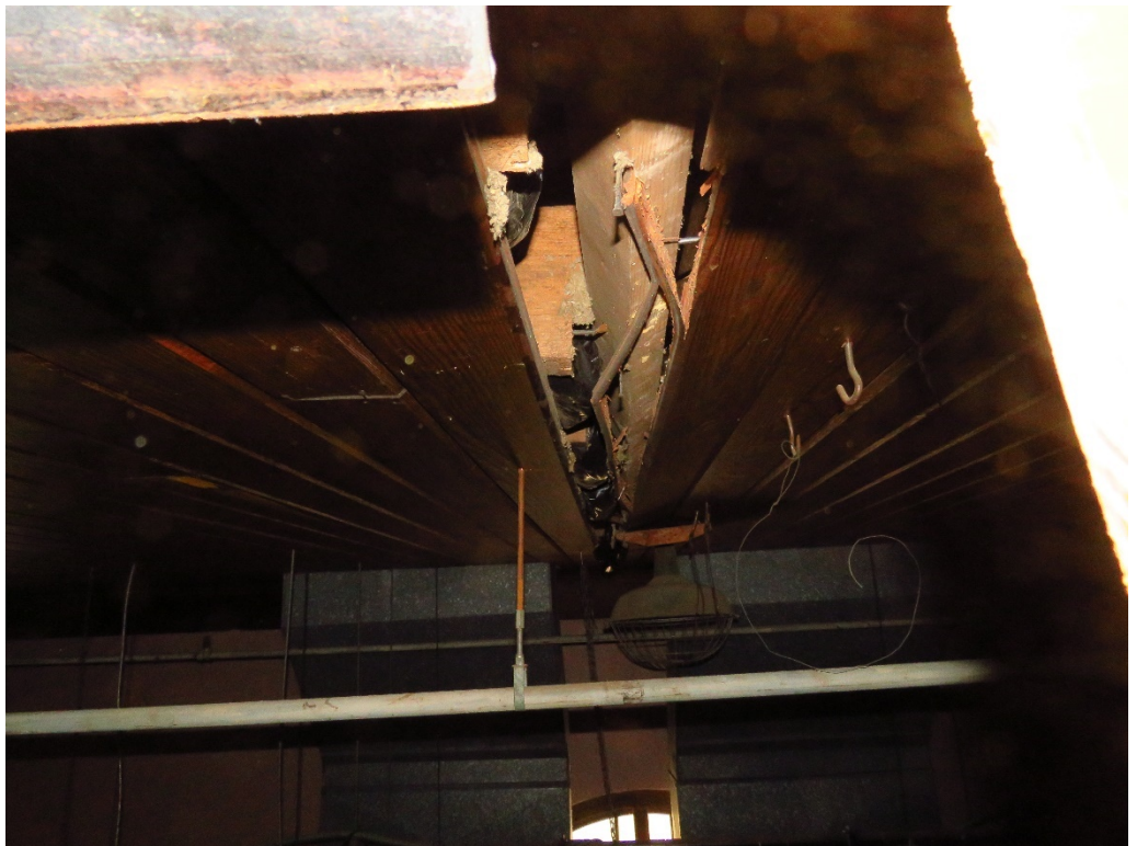
Figure 15: Ledger pulling away from north-south girder
