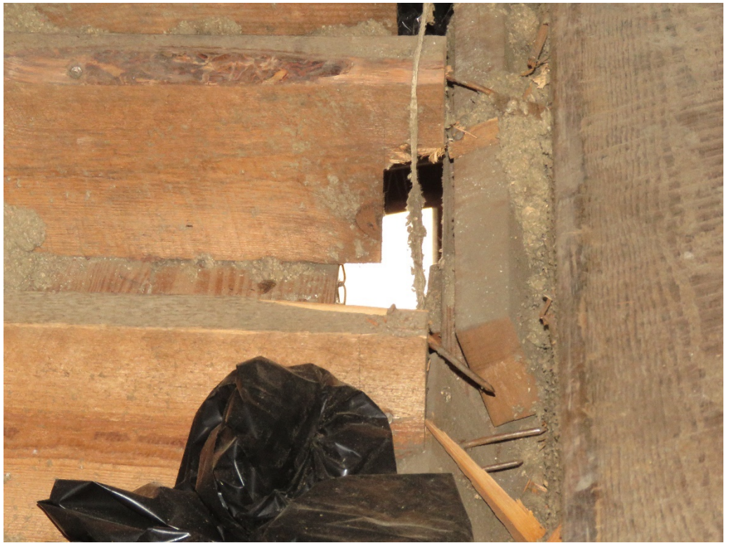
Figure 14: Ledger pulling away from north-south girder
