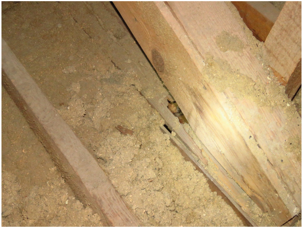
Figure 8: View of break in Truss1 from above
