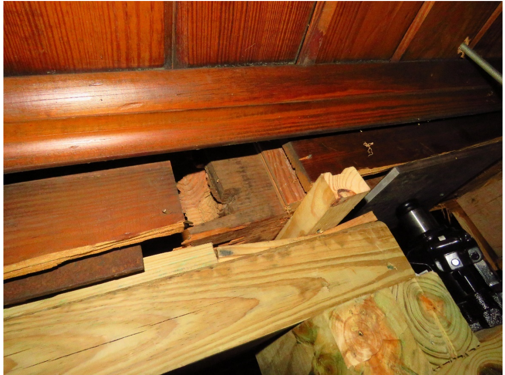
Figure 1: View of break in Truss 1 from below
