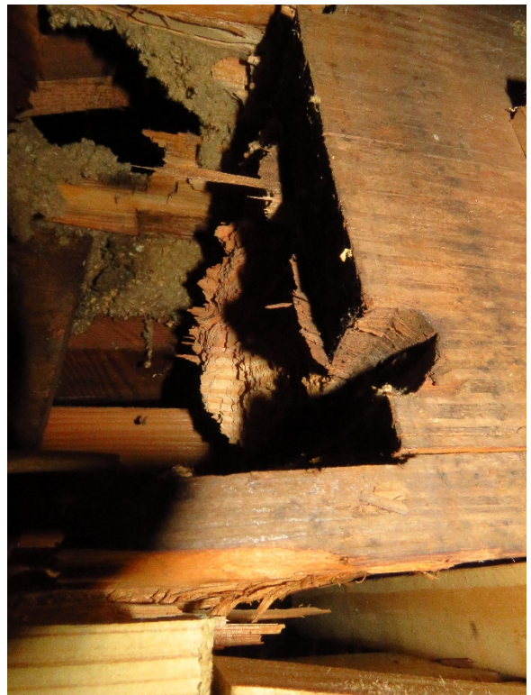
Figure 2: View of break in Truss 1 from below
