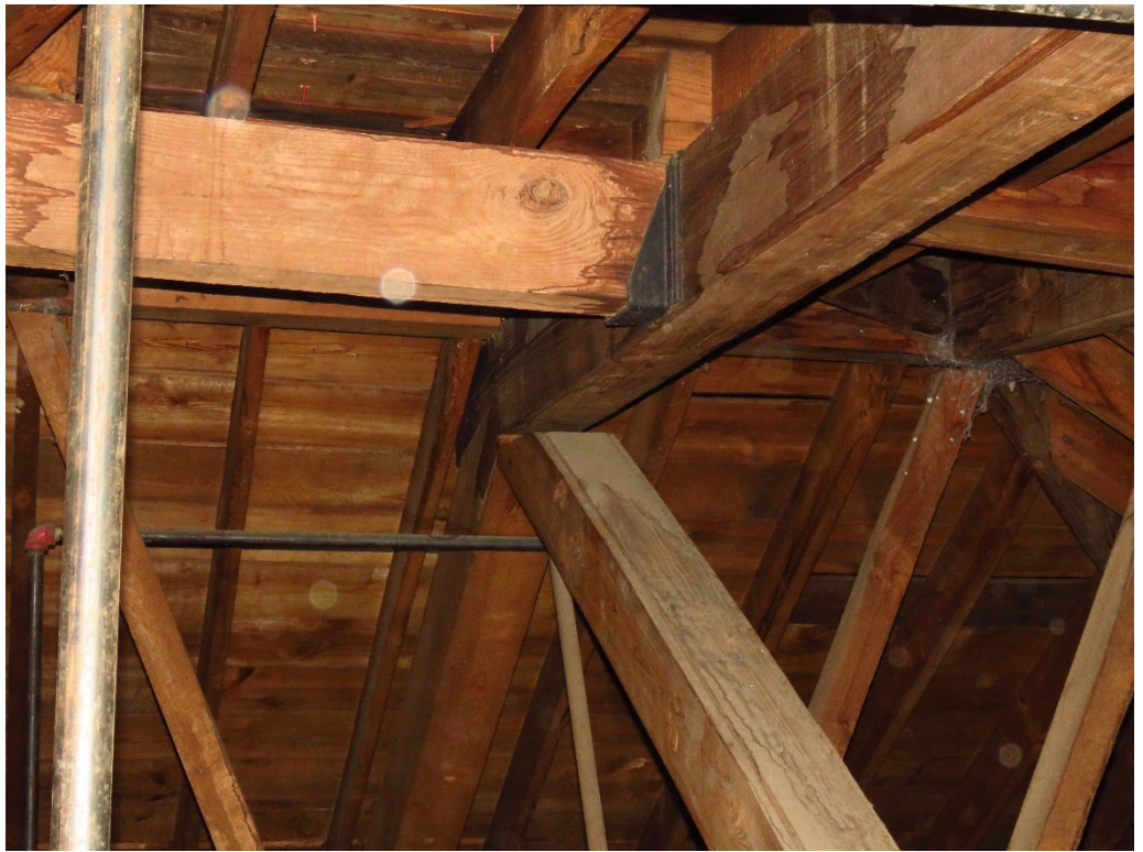
Figure 23: Disconnected diagonal at Truss 1
