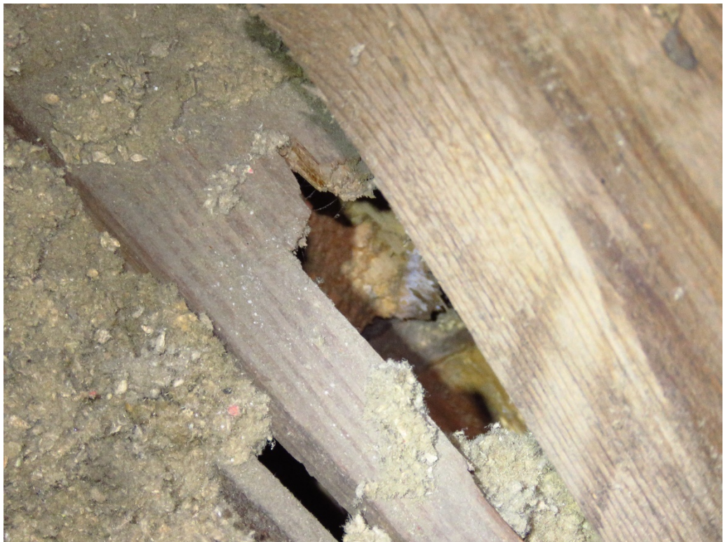
Figure 9: View of break in Truss1 from above
