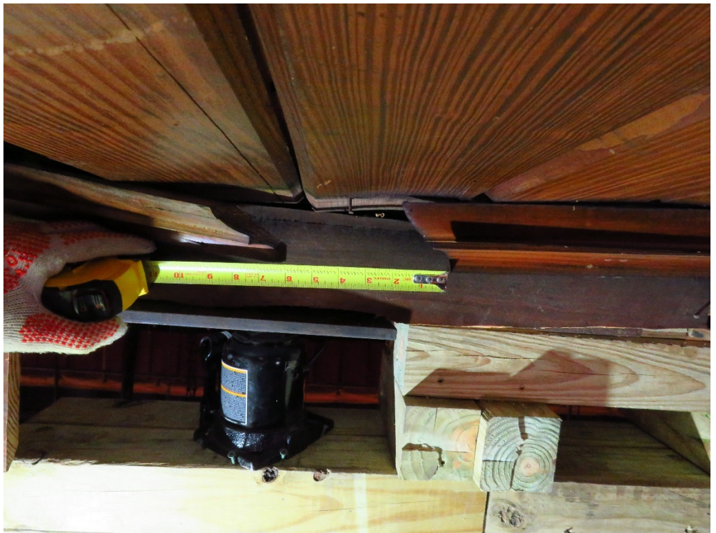
Figure 17: Open ceiling boards at Truss 1
