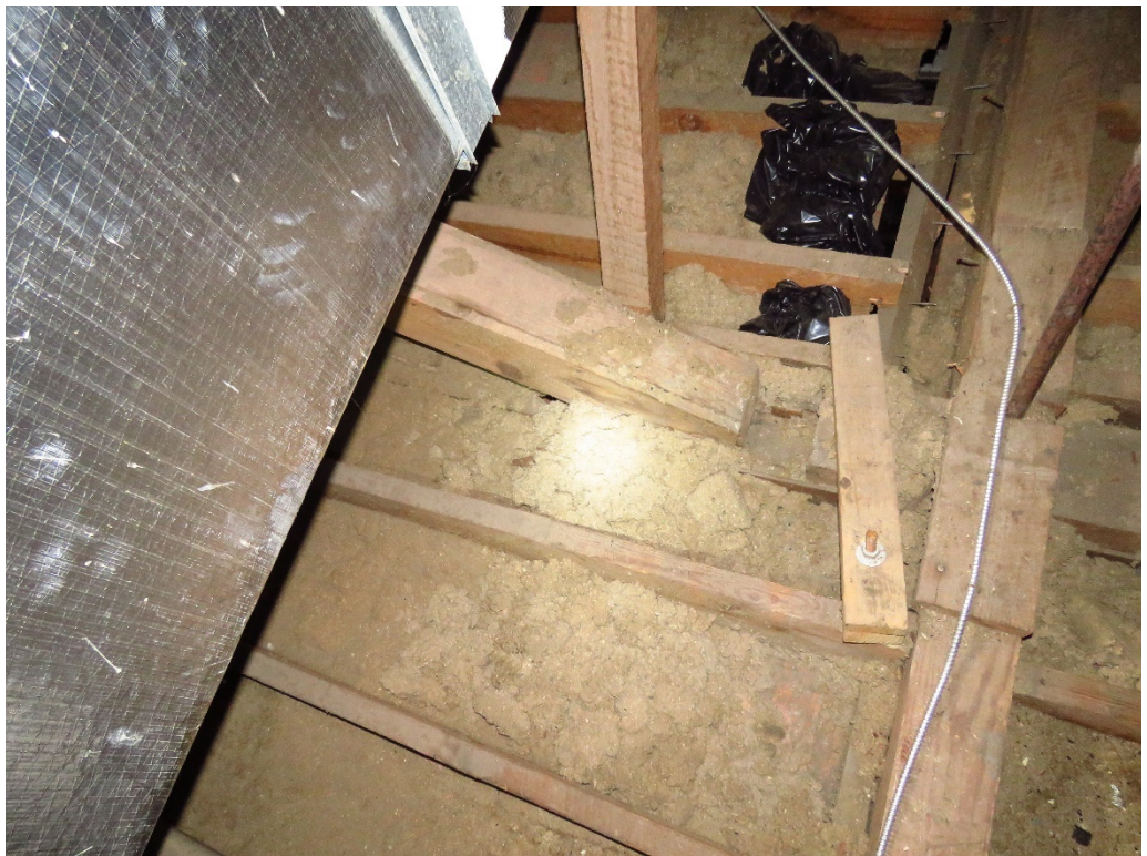
Figure 7: View of break in Truss1 from above
