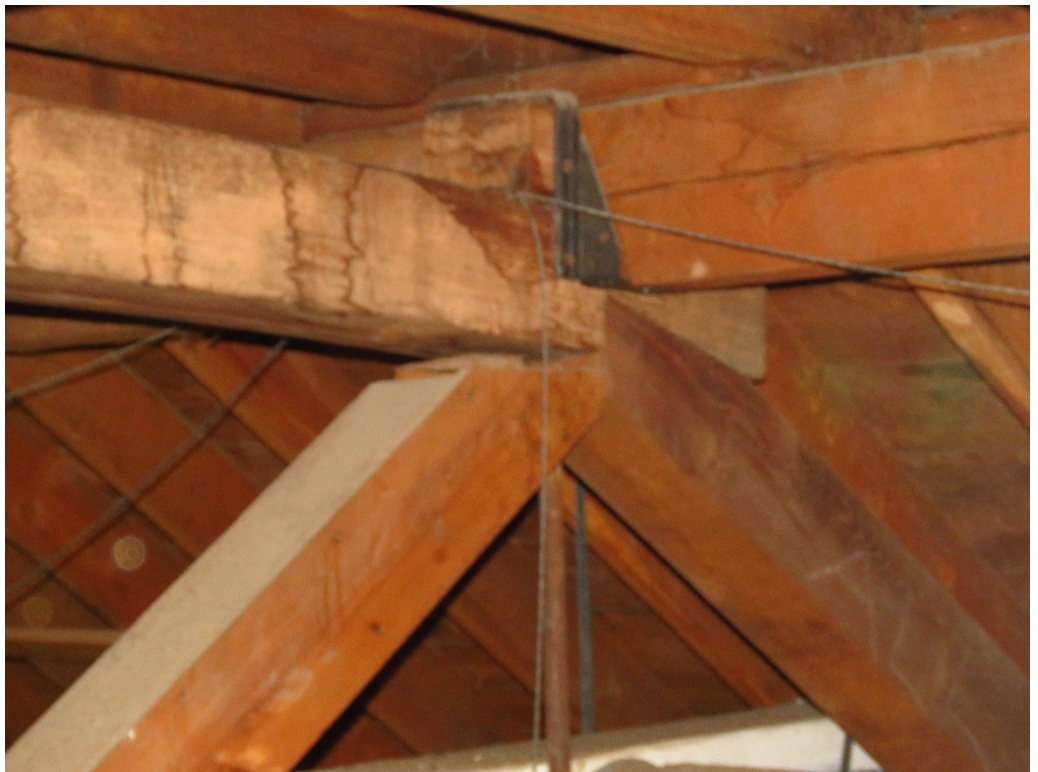
Figure 24: Disconnected diagonal at Truss 4
