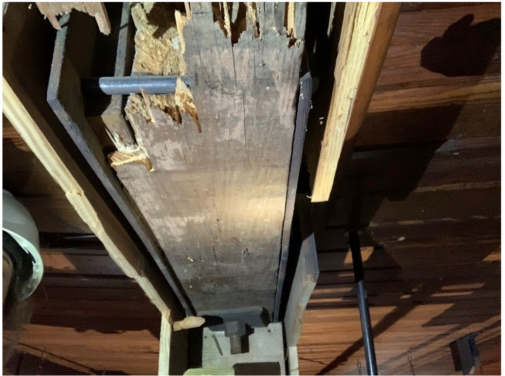
Figure 3: View of break in Truss 1 from below
