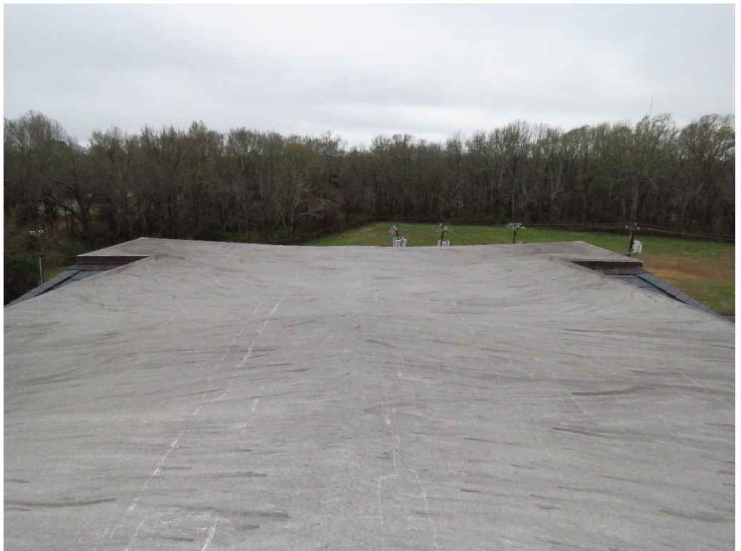
Figure 4: Condition of roof sag in March 2022
