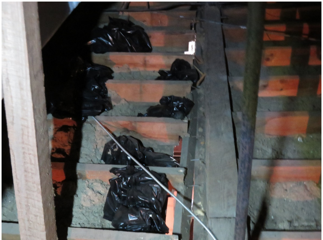
Figure 13: Ledger pulling away from north-south girder
